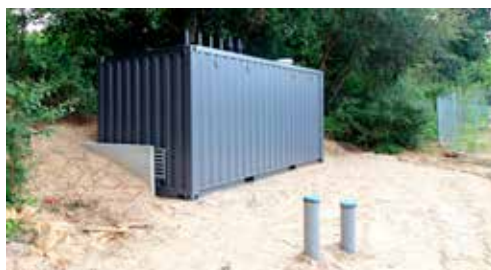
Verwarmingsunit in zeecontainer
